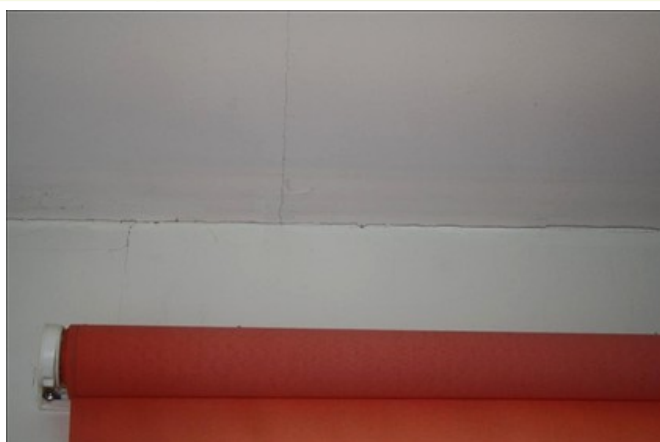
minor cracking where ceiling meets wall
