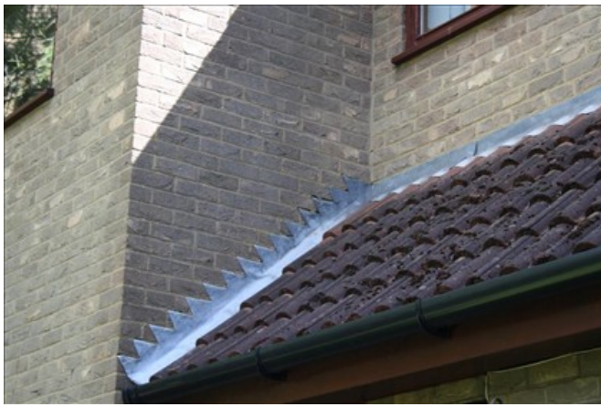
porch roof meets wall - some missing mortar
