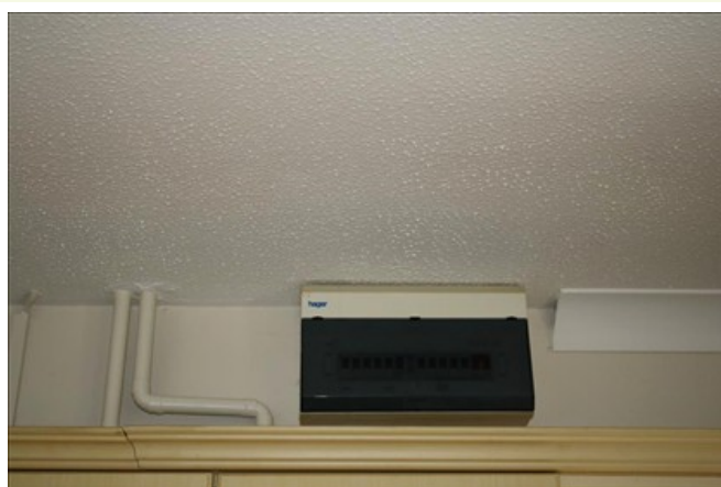
Consumer unit, above kitchen cupboard
