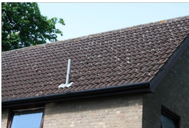
uncapped soil and vent pipe
