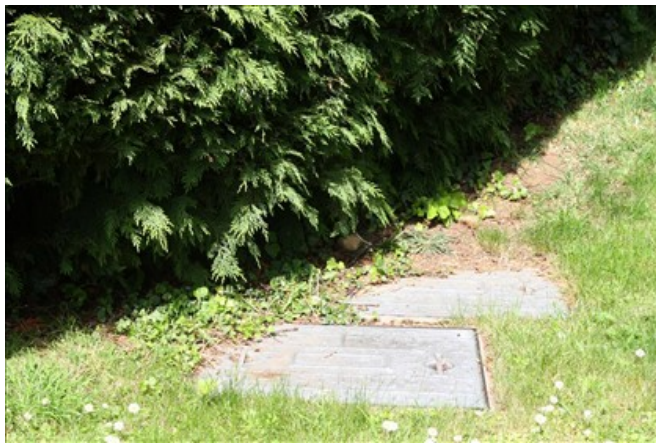
Inspection chambers not opened
