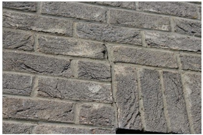
Crack to wall above patio doors
