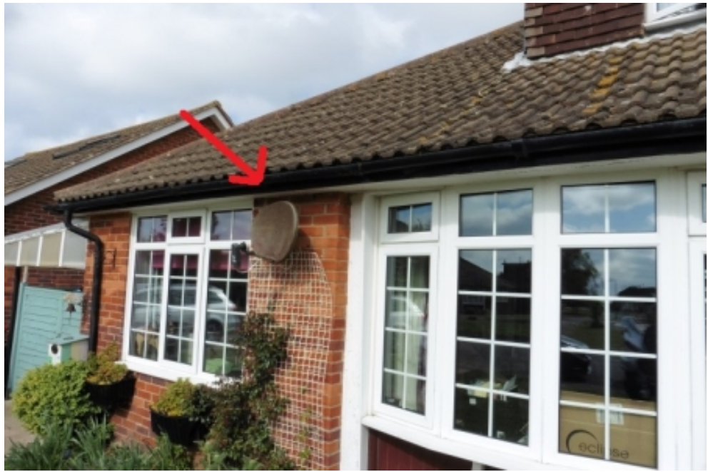
Sagging gutter at the front
