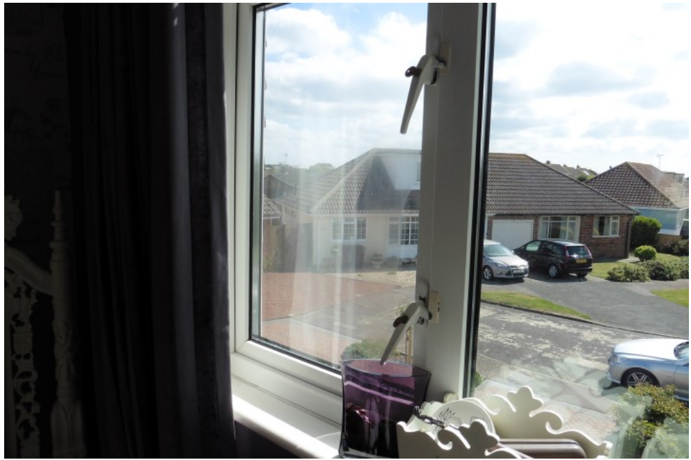
Bedroom 1 casement window panel blown
