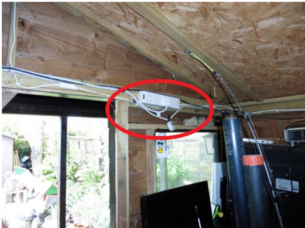
Poorly managed wiring in shed 4
