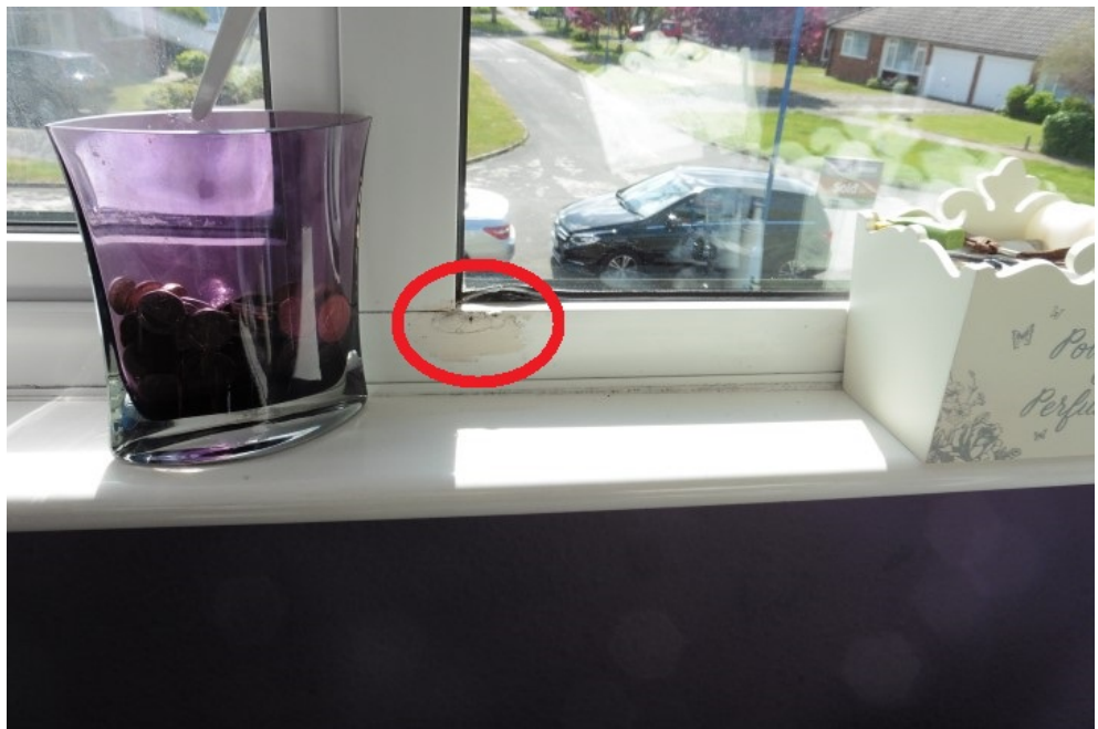
Damage to frame and seal in bedroom 1
