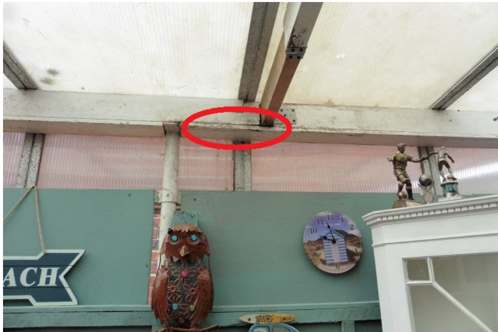
Possibly rotten timbers in the lean-to
