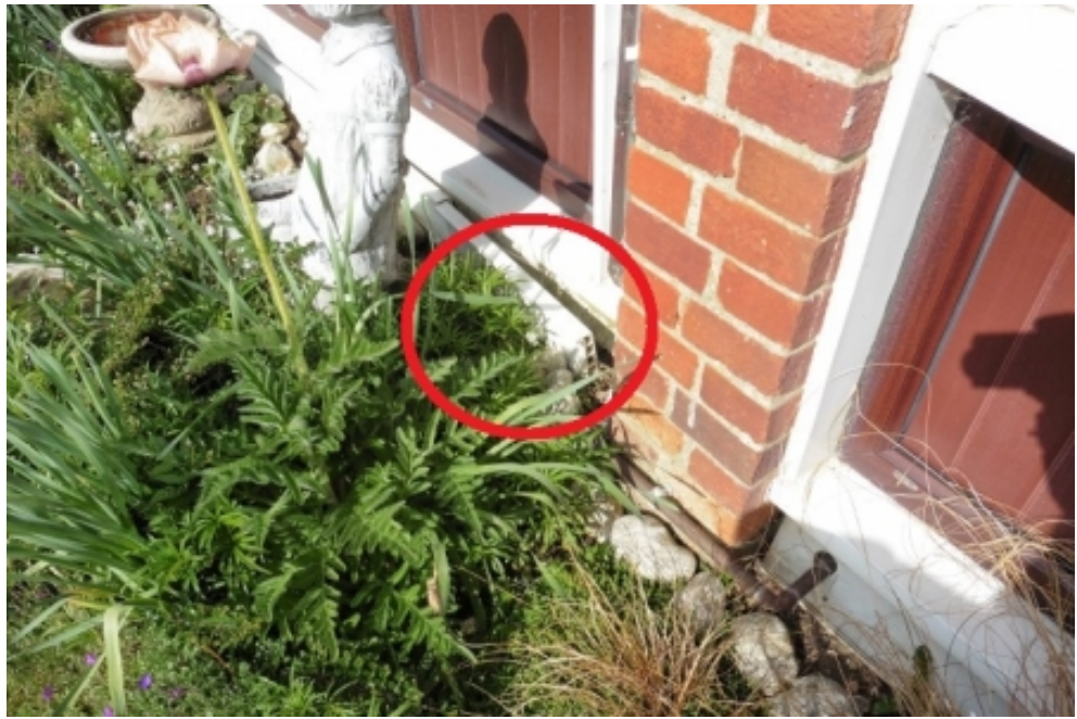
Loose plastic trim at the front
